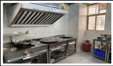
SS Exhaust Hood
