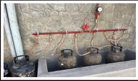
Gas Line manifold
